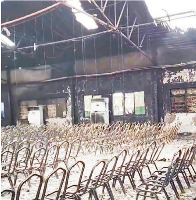
Debris of the church auditorium yesterday
